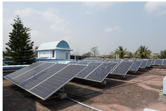
Figure 2.16. Solar Panel at the rooftop of Administration building
